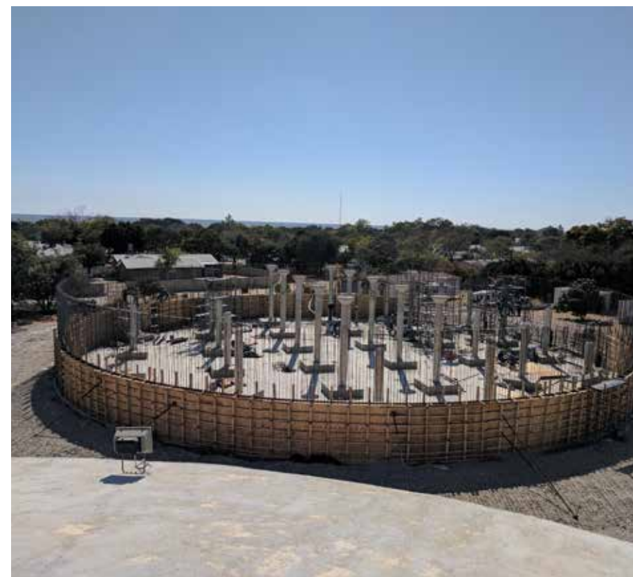
Nkarapanwe 12,000 cubic metre reservoir 2.
